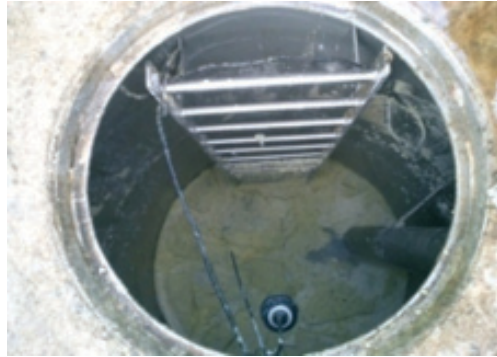
Grease build-up in wet well before EVOGEN G.T. treatment
